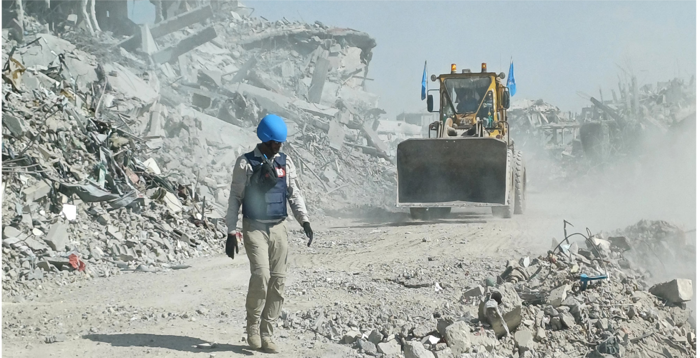
An Explosive Ordnance Disposal (EOD) Officer supervising and monitoring debris removal operations during a WFP-led road assessment, ensuring the detection and mitigation of potential explosive hazards. Gaza City, 18 September 2025 © WFP
